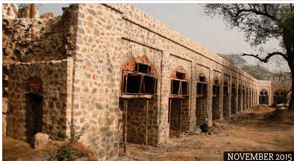
(Above) Collapsed portion of the Serai were carefully stabilized by master craftsmen building with techniques and materials used by the original builders.
